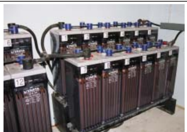
Figure 13 Figure 5-4. An off-grid system requires a means of storing the electrical energy generated by the renewable sources for later consumption. A sizeable battery bank provides the needed storage.
