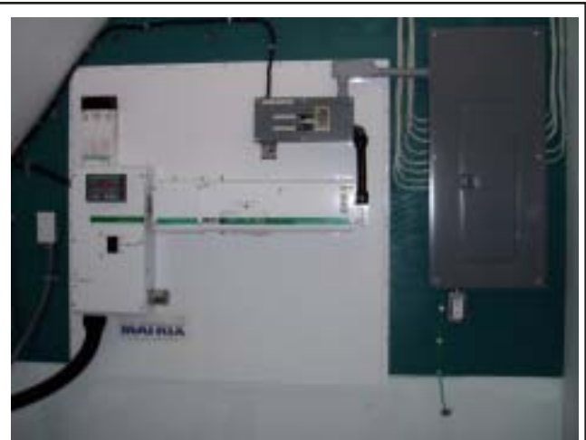
Figure 15. A renewable energy system should be neat, simple and well laid out, ensuring smooth sailing with electrical inspectors and your insurance salesman.
