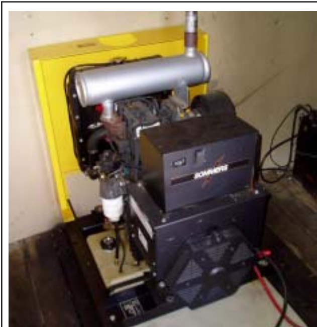
Figure 17. This large 7.5 kW diesel backup generator set (or genset) will last several lifetimes and be economical to operate as well.
