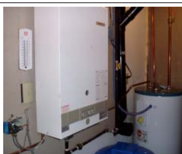
Figure 18. This home uses a high-efficiency, in-line gas water heater. The conventional storage water heater at rear is the diversion load, which absorbs waste energy by preheating the cold water fed to the gas water heater.
