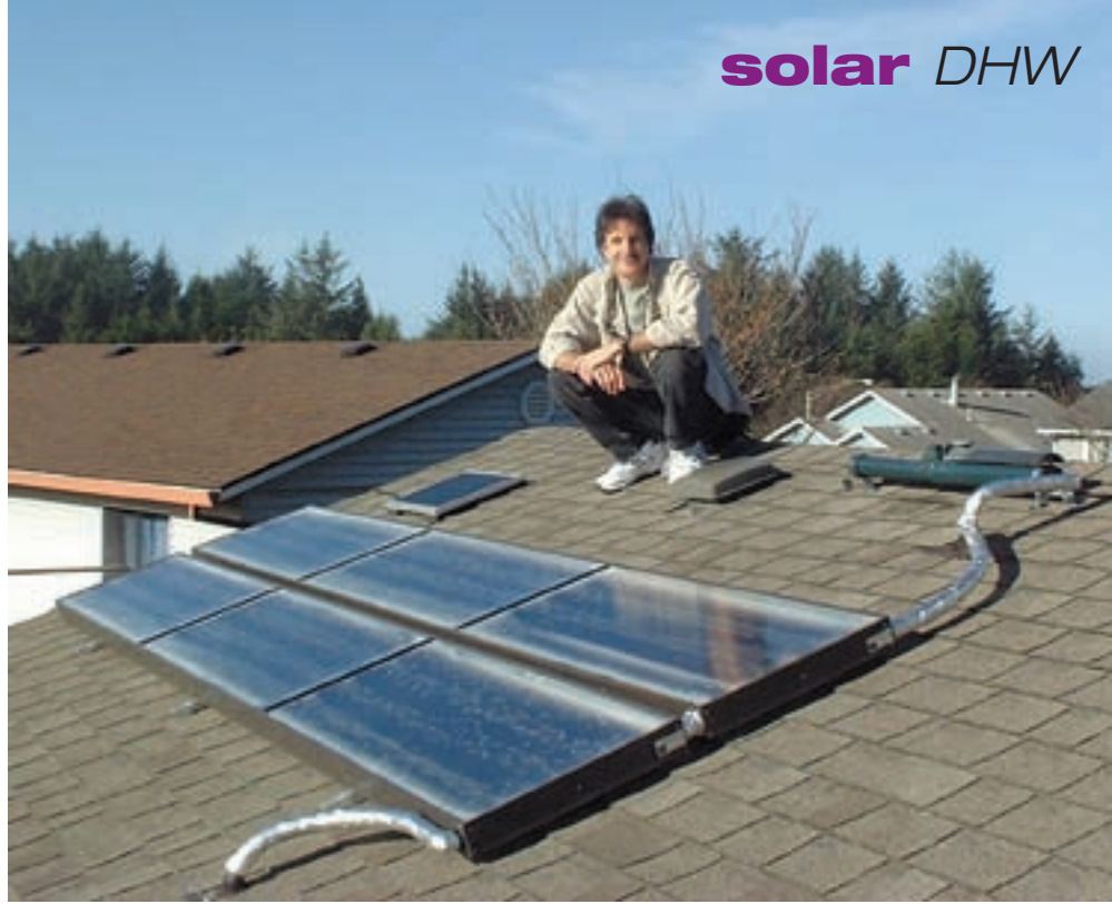
Solar installer Andrew Gerl of Blazing Solar of Mesa, Arizona, on the roof with solar thermal collectors, the PV module for the pump, and the TPFRS radiator/reservoir unit.
